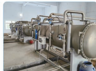
Gansu Lanzhou New Immigrant District Wastewater Treatment Plant Project
