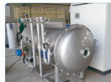
Anhui Langxi Dyeing and Printing Wastewater Treatment Project
