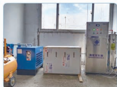
Shandong Dezhou Pharmaceutical Plant Sewage Treatment Project
