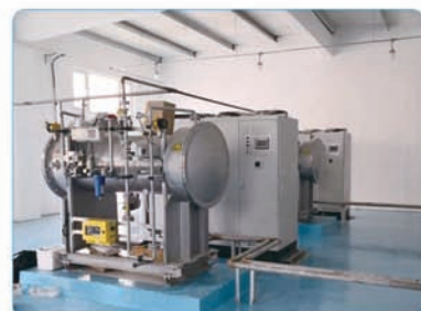
Hebei Gu'an Wastewater Treatment Plant Project
