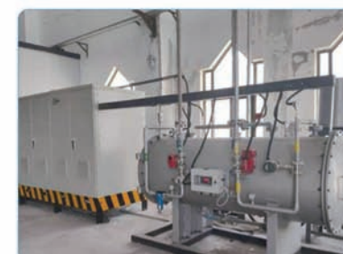
Hainan Haikou Bullfrog Farming Sewage Treatment Project
