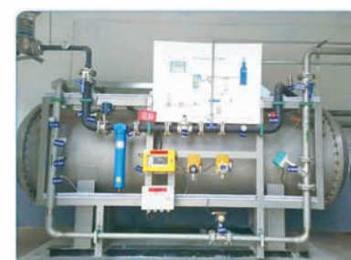
Medical Wastewater Treatment Project in Ili, Xinjiang
